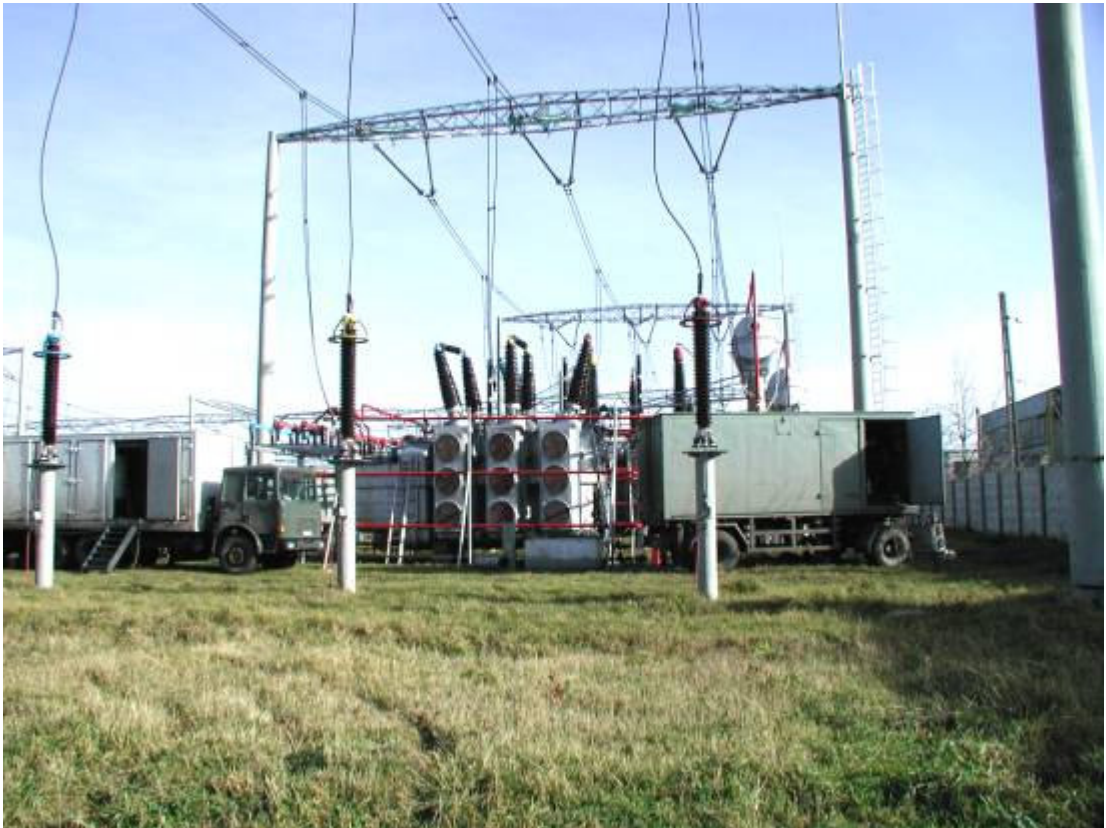
Photo 3: The insulation drying of (a+t) 400/60 MVA \pm [12 x 34,65/12] / 22kV regulating special transformer no. 85766/72, in 400 kV Sibiu-Romania substation
