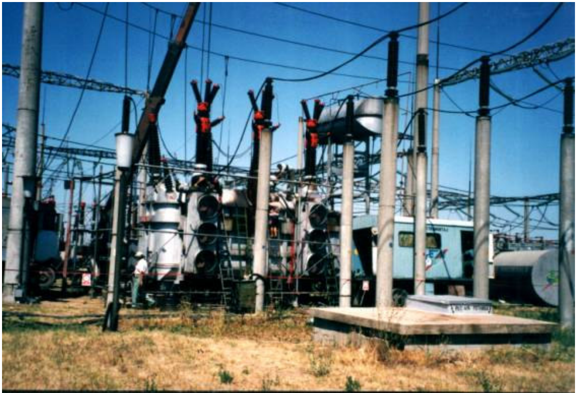
Photo 4. The insulation drying of 200/200/60 MVA 231\pm 8x1.56\% /121/20kV autotransformer no. 95731/1986, in 220 kV Turnu Magurele-Romania substation
