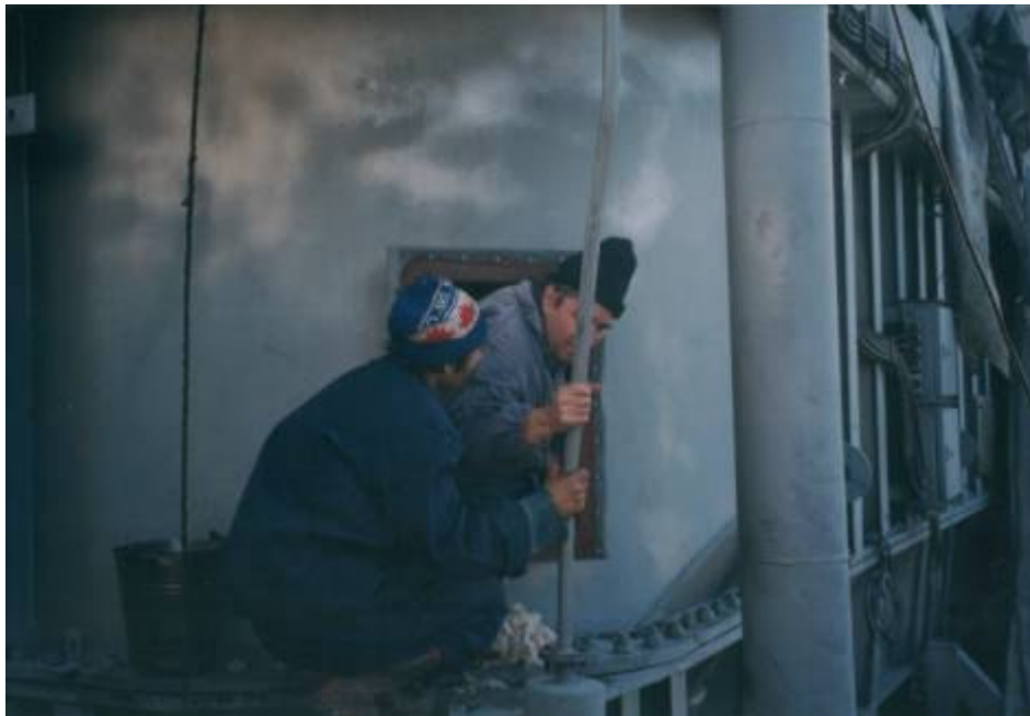
Foto 5 Entering of the Nova Industrial specialist inner of the 417/417/80 MVA 750 / \sqrt{3} / 400 / \sqrt{3} / 15,75 kV autotransformer tank, no. 128702/1986, to control and direct the activity of 525 kV failed bushing raising and its changing with a new one, in 750 kV Isaccea-Romania substation.
