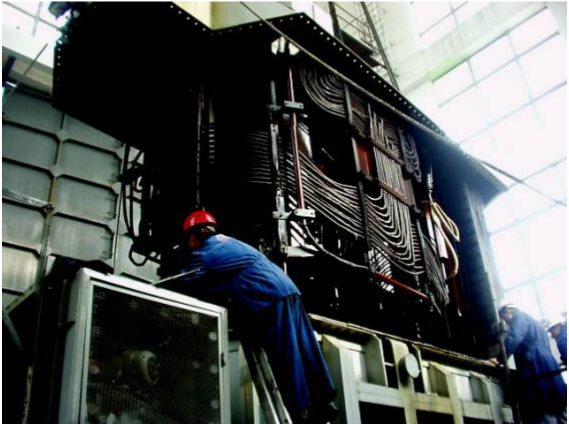
Photo 5: The control of active part of 66,6/66,6/21 MVA 231 \pm 12 \times 1,25\% / 121 / 10,5 kV autotransformer, no. 1173722/1966, in untanking tower, before insulation drying in 400 kV Iernut-Romania substation
