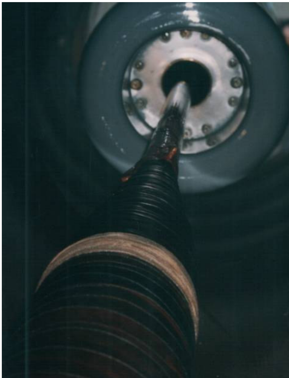
Foto 6 The control of 525 kV bushing raising from inner of the autotransformer tank
